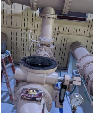
Figure 6: Typical check valve isolated and opened for inspection device insertion.
