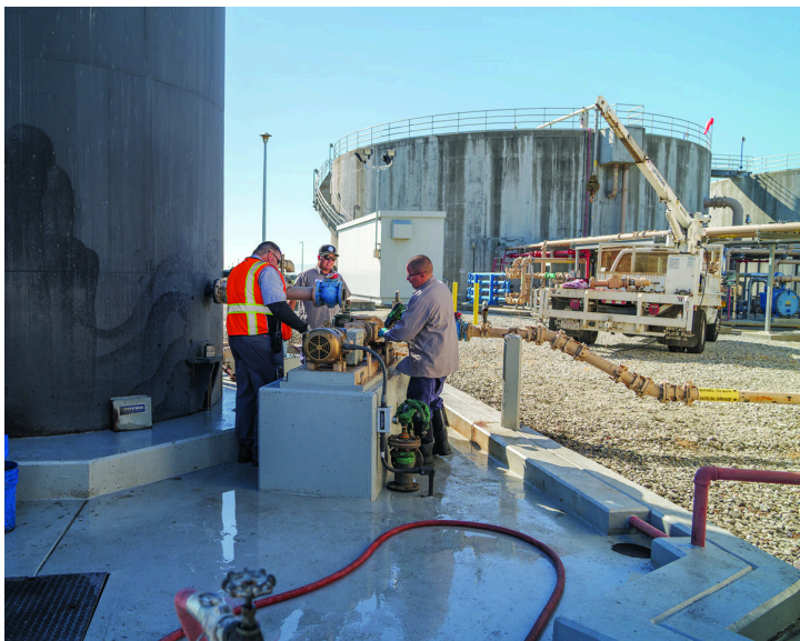
From left, Scott Beckman, operator, and Dallas Ledford and Jeff Hansen, mechanics, perform maintenance on a FOG receiving pump.
